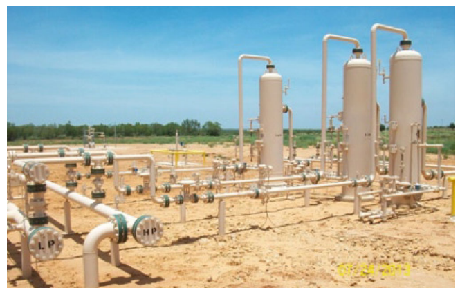
Emerson's 3-phase separator solution installed at the Eagle Ford Shale site
